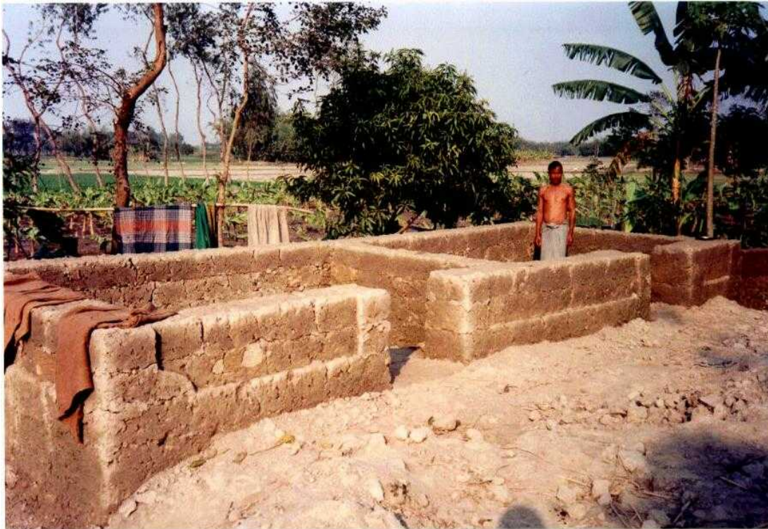
Photograph 13: A layered mud wall house under construction. This two-roomed house is being built by local builders whilst the householder is building his kitchen house himself. A decorative edging is incorporated into the carefully built walls.
