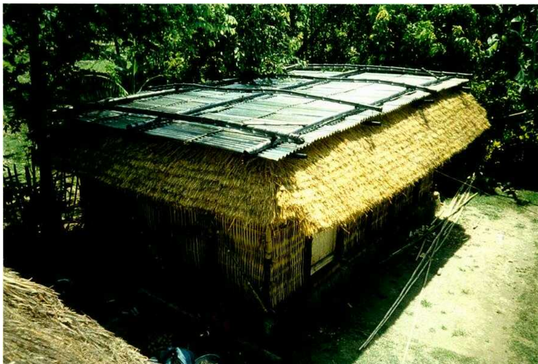
Photograph 10: The finished demonstration building: the bamboo frame for the sapra CI sheet roof has been painted with bitumen and lashed down with strong wire.
