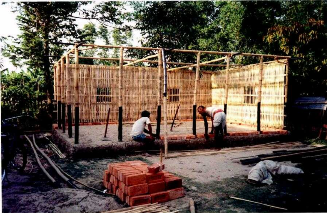
Photograph 9: The demonstration building under construction: laying a proof course to protect the walls from rot and insect attack.
